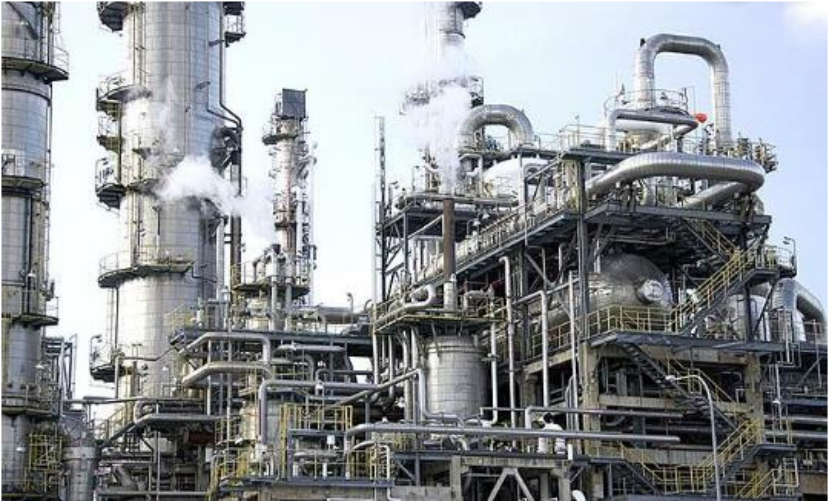
Oil refinery catalytic reactor
